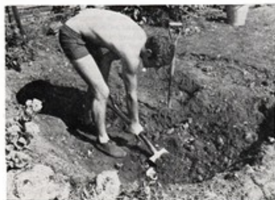
After the excavation has been made of the size required the hole should be lined with discarded plastic or paper to form a thick pad between the 500 gauge sheeting and the soil
