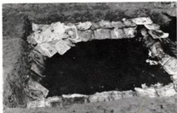
After completion of the shaped excavation its base is covered with sedge peat and the sloping sides are covered with damp newsprint to cushion the liner
