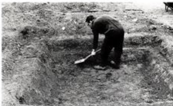
Final stages of the excavation involve the shaping of the sides. These must slope inwards so that no vertical parts to the sides occur
