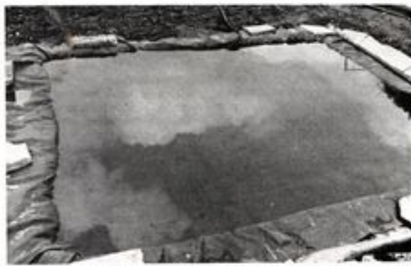
With the liner in position in the hole, stone slabs are placed around its overlap to keep the top edges in position during the filling with water
