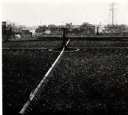
The rotating arms of this sewage filter system deliver jets of the sewage on to a bed of clinker. Biological purification occurs as the water percolates through the bed
