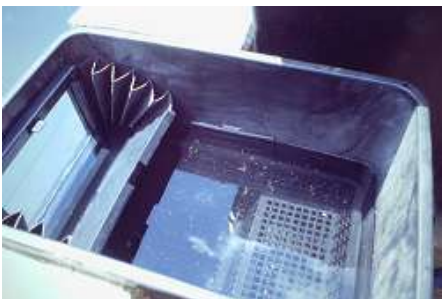
11. Inside skimmer (workings).
