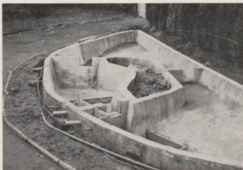
Koi pond under construction showing island and three separate compartments which can be isolated from each other by water-tight gates.
