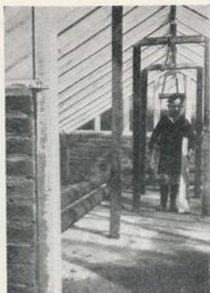
Clearing the house interior before construction of concrete tanks and before glazing is complete. The heating pipes are seen in position.
