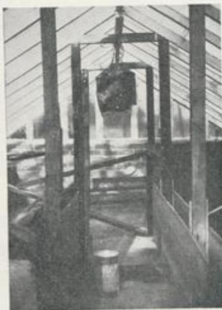
Shuttering for the concrete tanks to be made inside the house is shown ready for the pouring of concrete
