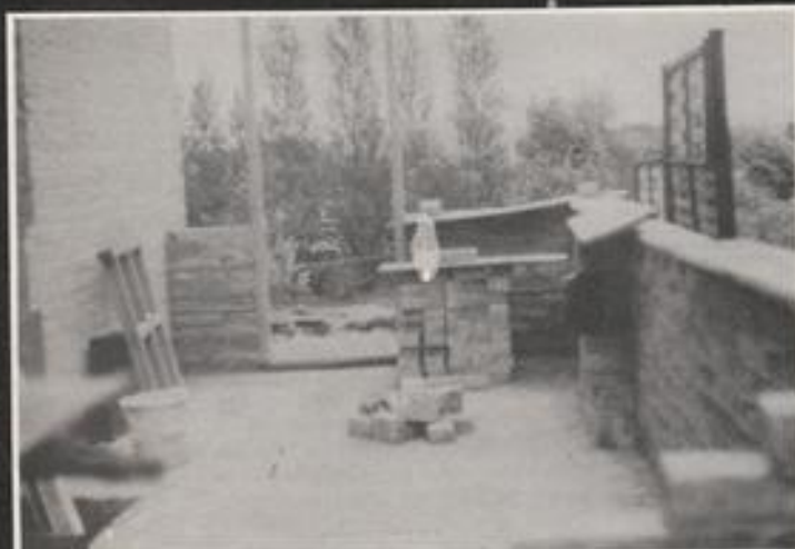
Photograph 1 shows the project at a stage when the brick laying is about one third complete. Note the position of the block wall two thirds of the way from the front wall
