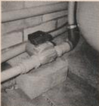
Showing the reduced pipework connected to the pump with PVC fittings
