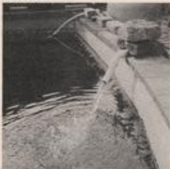
In the far corner can be seen the suction pipe connected to an under-gravel filter, and in the foreground showing about 800 gallons/hour return from the pump
