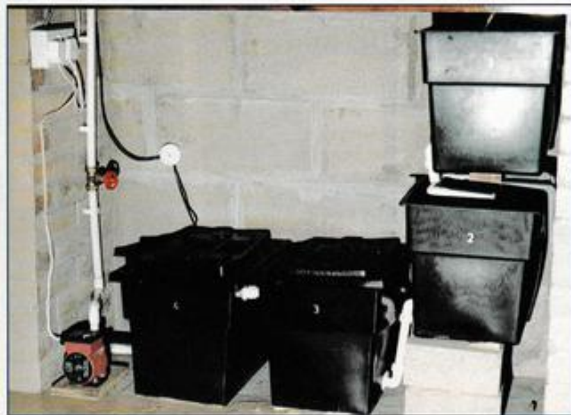
Close-up of three stage filter.
