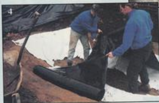
5 As the pond fills with water, pleat the liner to minimise creases and mould into contours.
