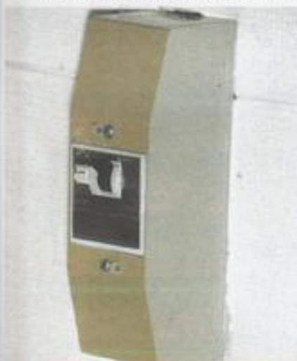
An RCCB (circuit breaker). This is mounted on the wall in the kitchen and the electrics to the whole garden are run from it.
