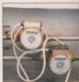
My faithful, long-running Grundfos pumps are housed in a waterproof chamber.
