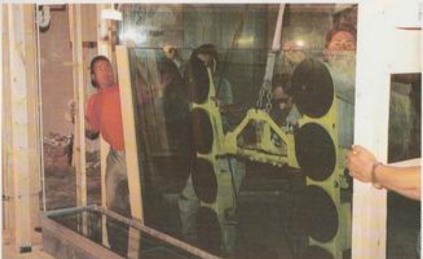
Lifting one of the 18, 1000-lb sheets of toughened glass into position. See next month's A&P for all the details.
