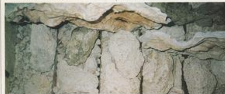
The back wall and overhang (right at the top of the shot) nearly completed.
