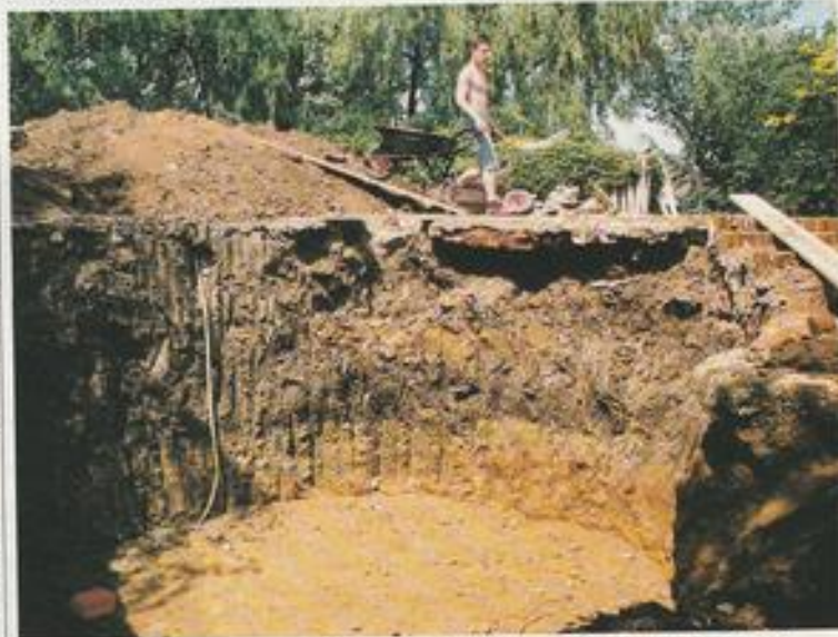
Excavations as deep as this should have a perimeter demarcation to prevent accidents.
