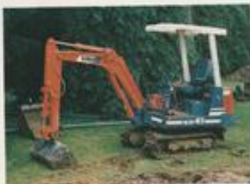
For large excavations it's well worth considering the hire of a digger.
