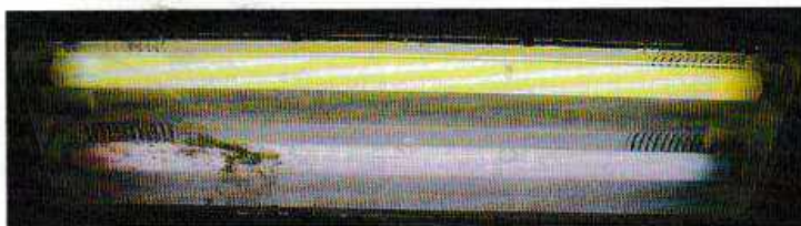
Keeping your light tubes clean and replacing tubes every year will ensure the best possible output
