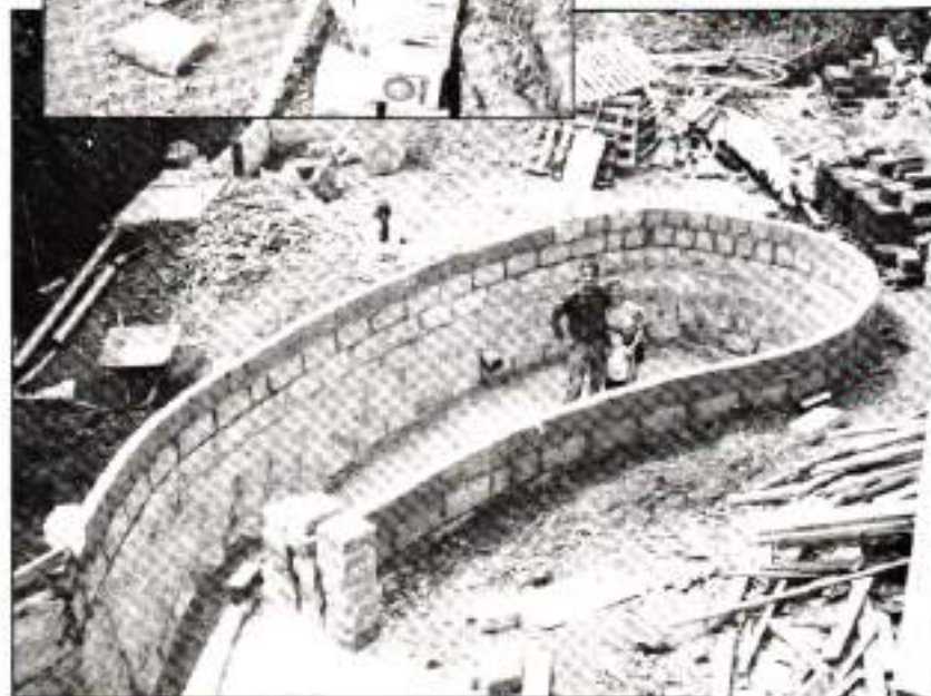
Below: The pond takes shape. Gravity intake to the filter (wing built top left) is visible.
