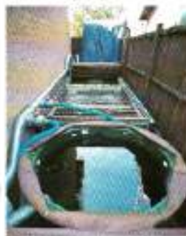
The filter system is outside the house.
