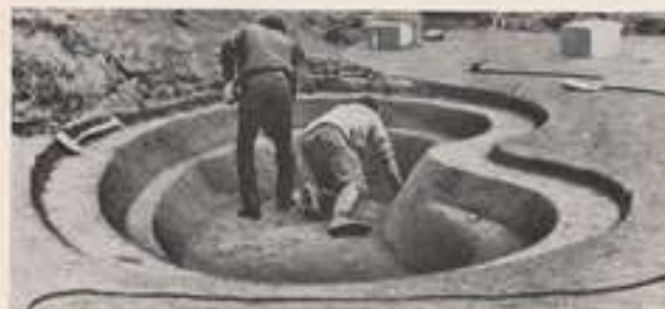
Making the excavation: turf has been removed for 24 in. beyond the pool outline for paving stone edges to be laid level with the lawn. Stones are removed and sand laid on the base and sides.
