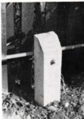
Conduit protects and carries cable to the fish house above ground on concrete posts
