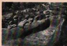
The bottom pond covered and rendered with the lower layer of artificial rocks completed.
