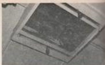
Main ventilator housing the air extractor
