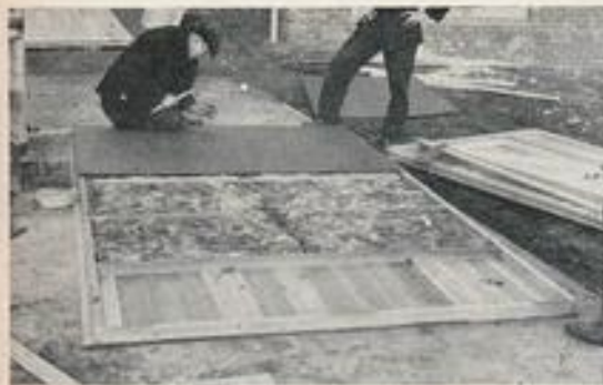
One of the long wall sections (10 ft.) made of red cedar wood is seen being packed with glass wool and covered on the inner side with hardboard before erection. The cavity nearest to the camera is seen without its glass wool
