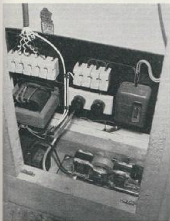
Electrical equipment beneath the aquaria of the fish-room unit is reached by removal of one of the lower panels
