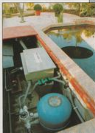
904 Model installed on pond of 4,200 gallons
