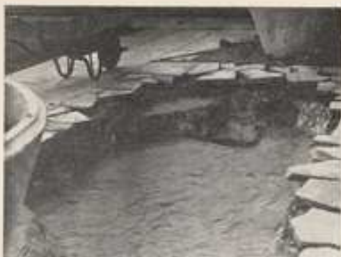
Above: The excavation with sand-layered base ready to receive the plastic sheeting
