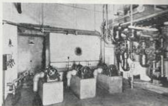
Filtering and pumping equipment in a large public aquarium —the famous Shedd Aquarium in Chicago, U.S.A.
