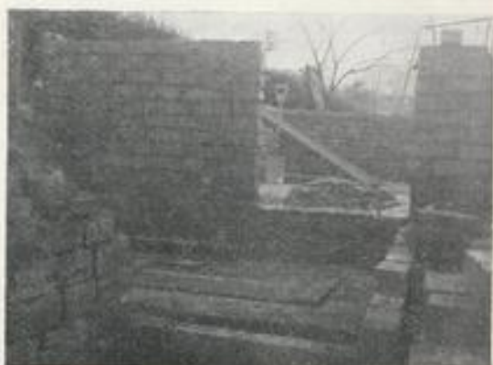
The building at a stage during the construction of the "boiler house"
