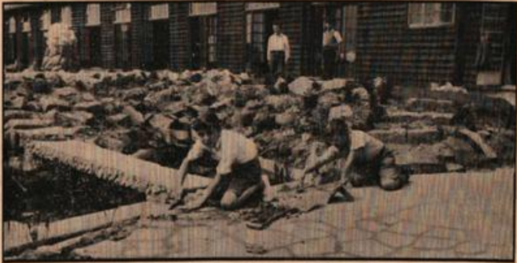
Fig. 6 (above) shows one of the final stages of this most excellent job of work. The pool has been satisfactorily tested, and found to be watertight. A few plants have already been established, and the crazy paving approach is being finished off. Note the obvious youth of the "labourers."
