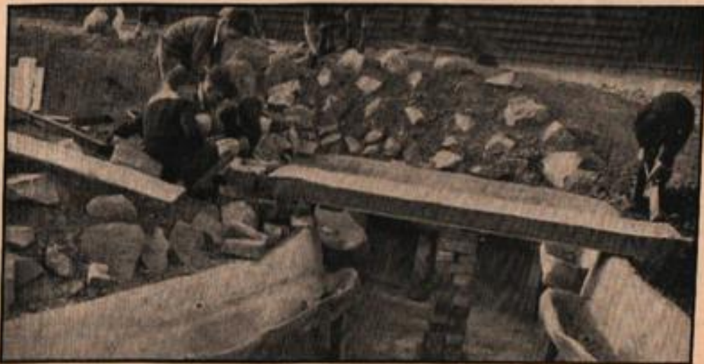
Fig. 4.—Here the sides have been rendered, and the planting troughs constructed, while a narrow bridge has been added, and is seen being supported by a pile of bricks during the hardening process.
