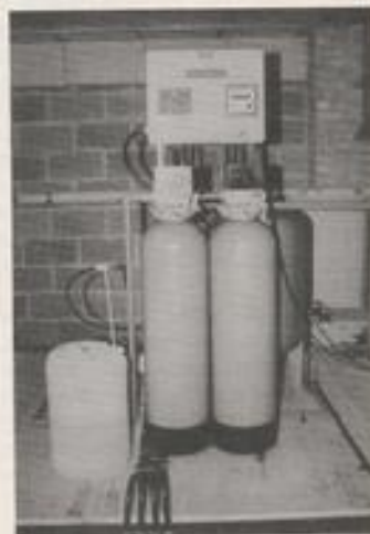
Resin-filled pH water treatment cylinders
