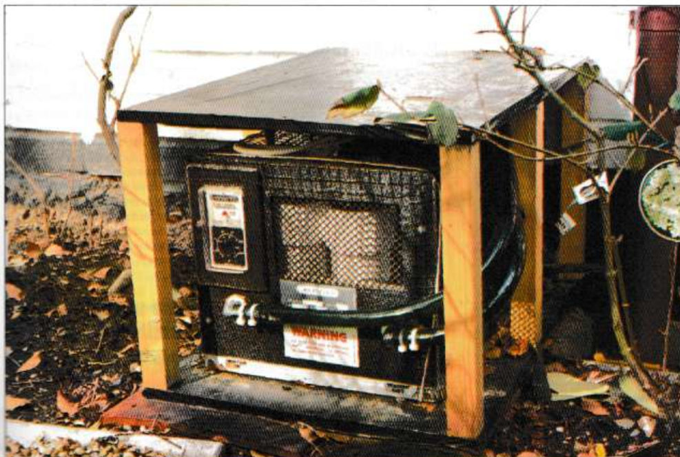
Aquarium chiller properly situated outside.
