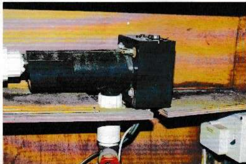
An electric swimming pool heater plumbed in line with return to pond.
