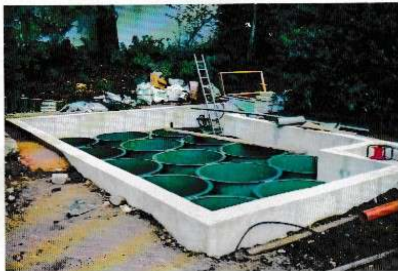
A total Vortex filter system.
