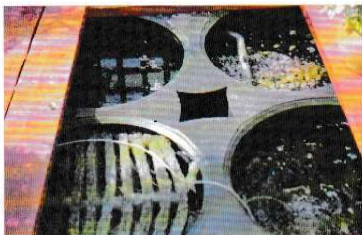
Filter system for Koi pond.
