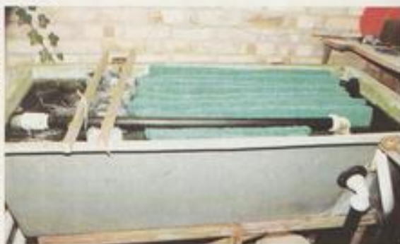
A filter system using brushes and matting to service a quarantine system.
