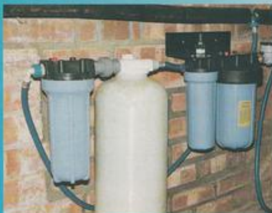
Water purifier mounted in an ideal position, in a garage near to the central heating boiler (but not too near!). It is fed from the owner's old dechlorinator unit as mentioned in the text. Note that this keeper has also got a water meter fitted which will give him an indication of when the cartridges are approaching exhaustion.
