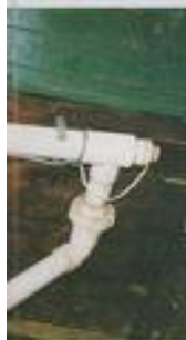
A UVS on a pond system. If installed outdoors, as this one is, it is important to ensure that it is rainproof.
