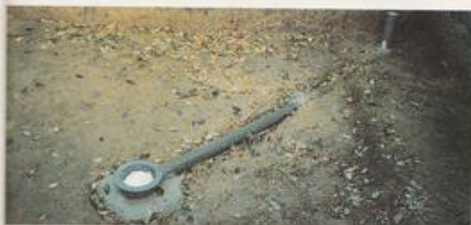
The installation of a bottom drain is very important for an efficient Koi pond filtration system.
