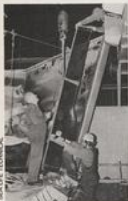
Technicians of Sea Life Centre Technical re-align the new window panes of the giant display aquarium at Kingdom of the Seas Aquarium, Hunstanton.
