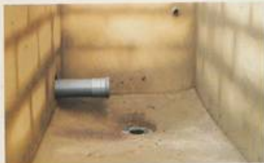
Filter chamber under construction showing the inlet from pond wall drain. The bottom outlet drain will be opened periodically to remove accumulated waste.
