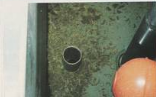
This photograph shows the efficient waste collection (at the settlement stage) of a well designed gravity-fed filtration system.
