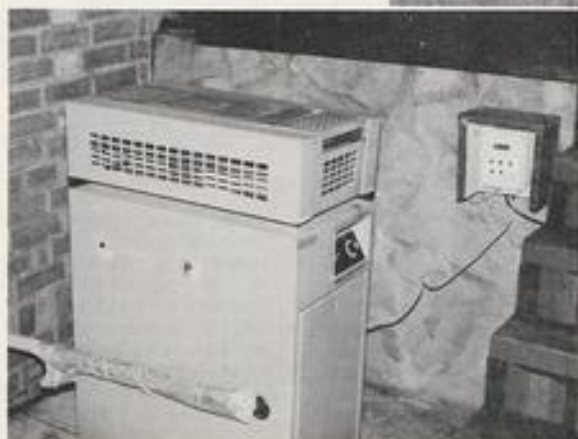
A typical gas boiler installation.
