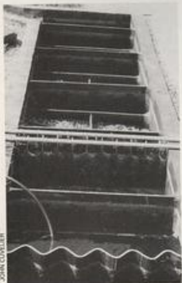
A sunken home-built concrete/Fibromix multi-chamber filter.
