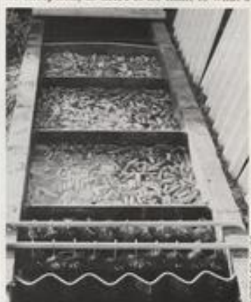
My below-ground gravity fed multi-chamber filter. Note the two rows of brushes for pre-filtration.
