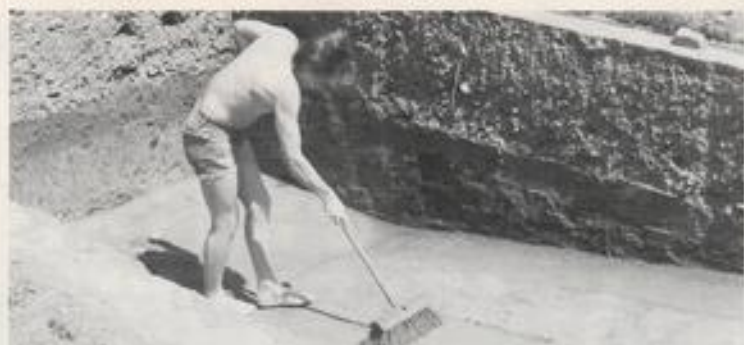
No. 1 son, Alex, preparing the ground to receive its carpet prior to fitting polystyrene sheeting around the walls and then fitting the butyl liner.
