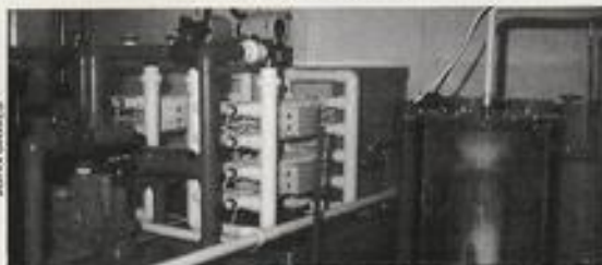
Hambridge's brand-new and impressive water treatment room.
