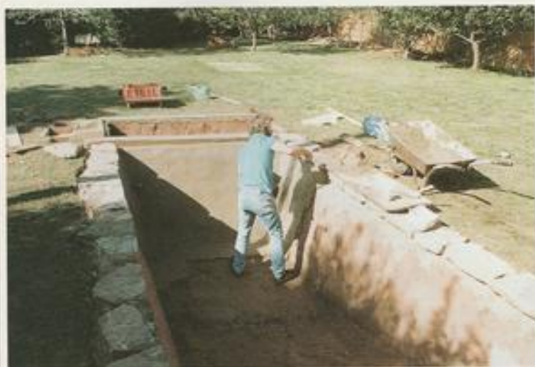
Rendering of the newly-dug 'hole' well underway. Note the filter chamber at the far end.
