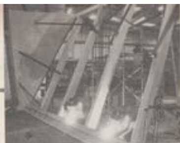
Viewed from inside the tank welders work on the giant sloping front of the aquarium
