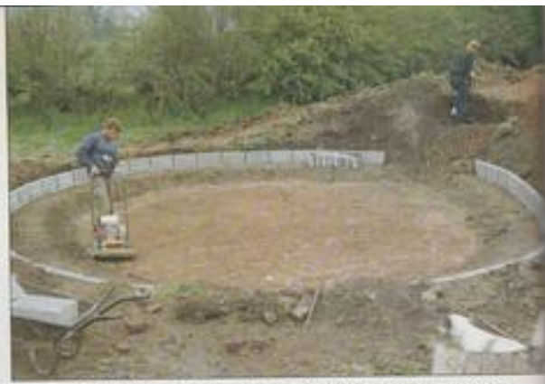
A 'whacker plate' is a tremendous help when it comes to flattening and compacting loose sods and bits of grit.
