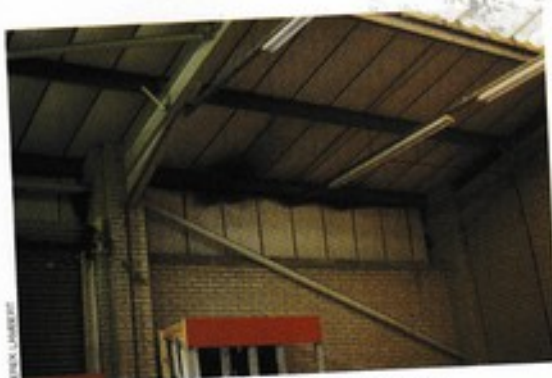
● The last traces of smoke damage that caused so many problems.
